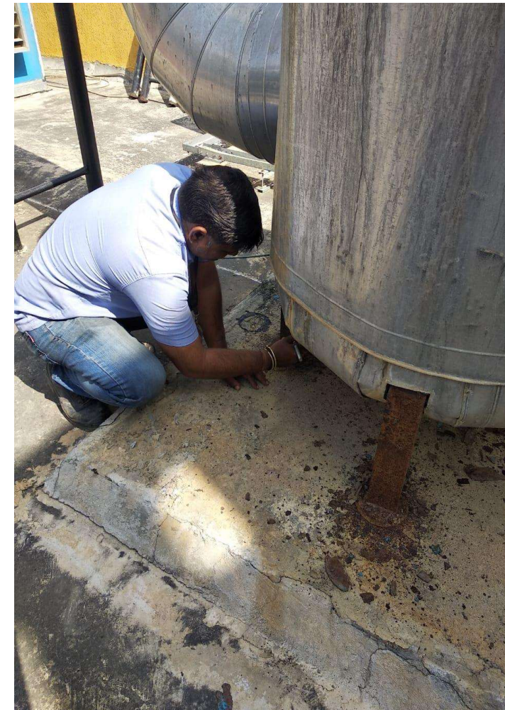
Expansion Tank Cleaning – 2 AB
